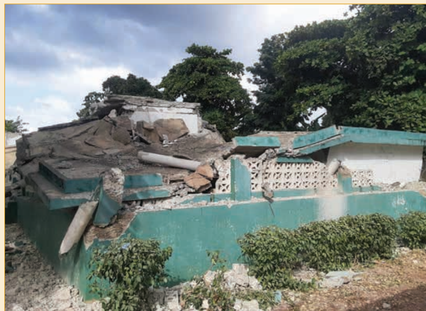
Wreckage of a clinic at our Haiti South site.
